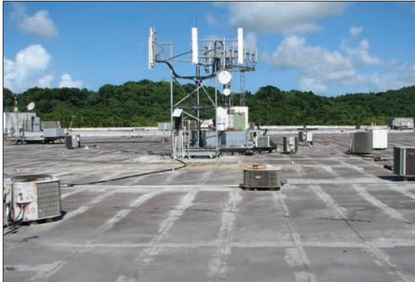
Corrosion (rust) in view of the antenna can cause PIM
