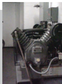
Air Compressor – Full Visible
