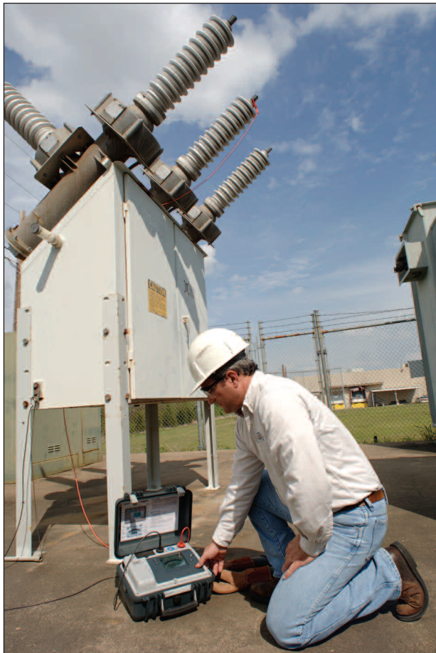
The MIT1020/2 in use at an industrial complex substation
