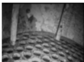
Corrosion of heat exchanger end plate
