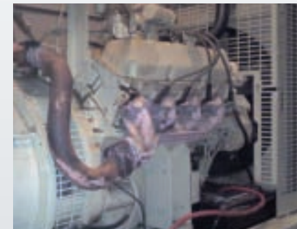
Visual Image of Generator
