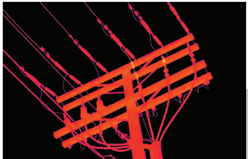
Electrical utility distribution lines
