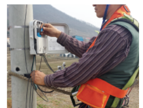
WORK BELT On a Telephone pole
